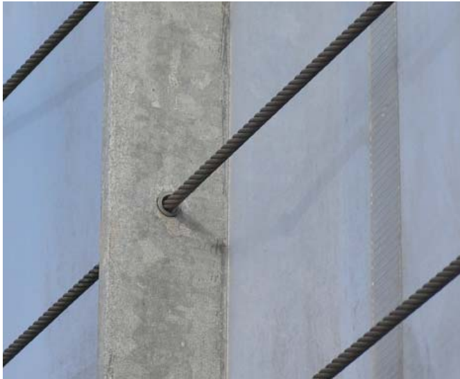
Use of plastic inserts prevents dissimilar corrosion between stainless steel and galvanized steel in coastal environment
