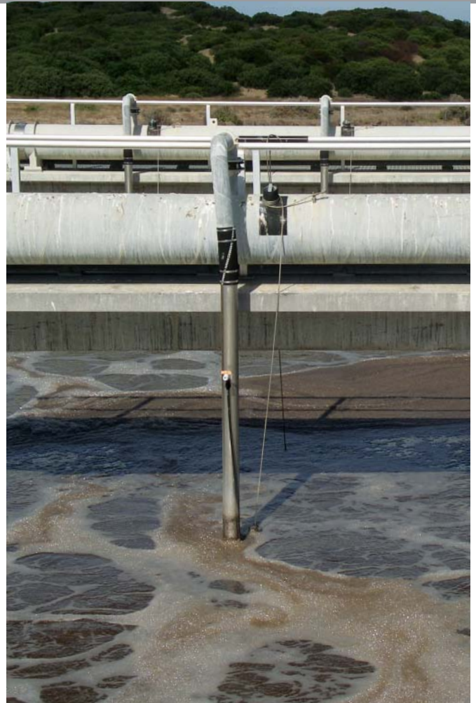
Galvanized pipes carrying air to aeration tanks
