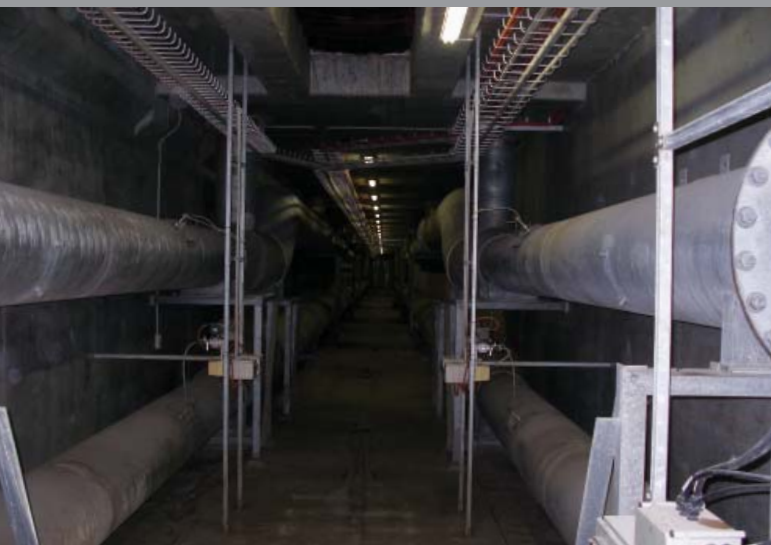
Underneath the facility - Galvanized pipes carrying air to aeration tanks
