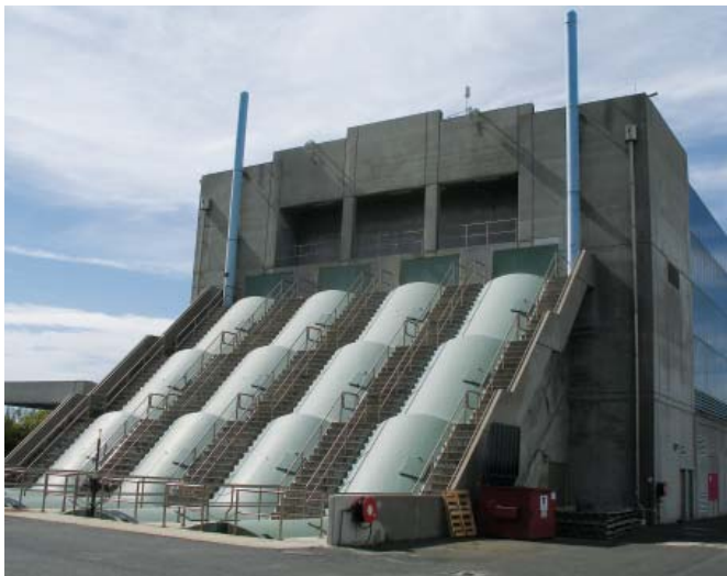
Archimedean screws carrying sewage to milliscreening plant
