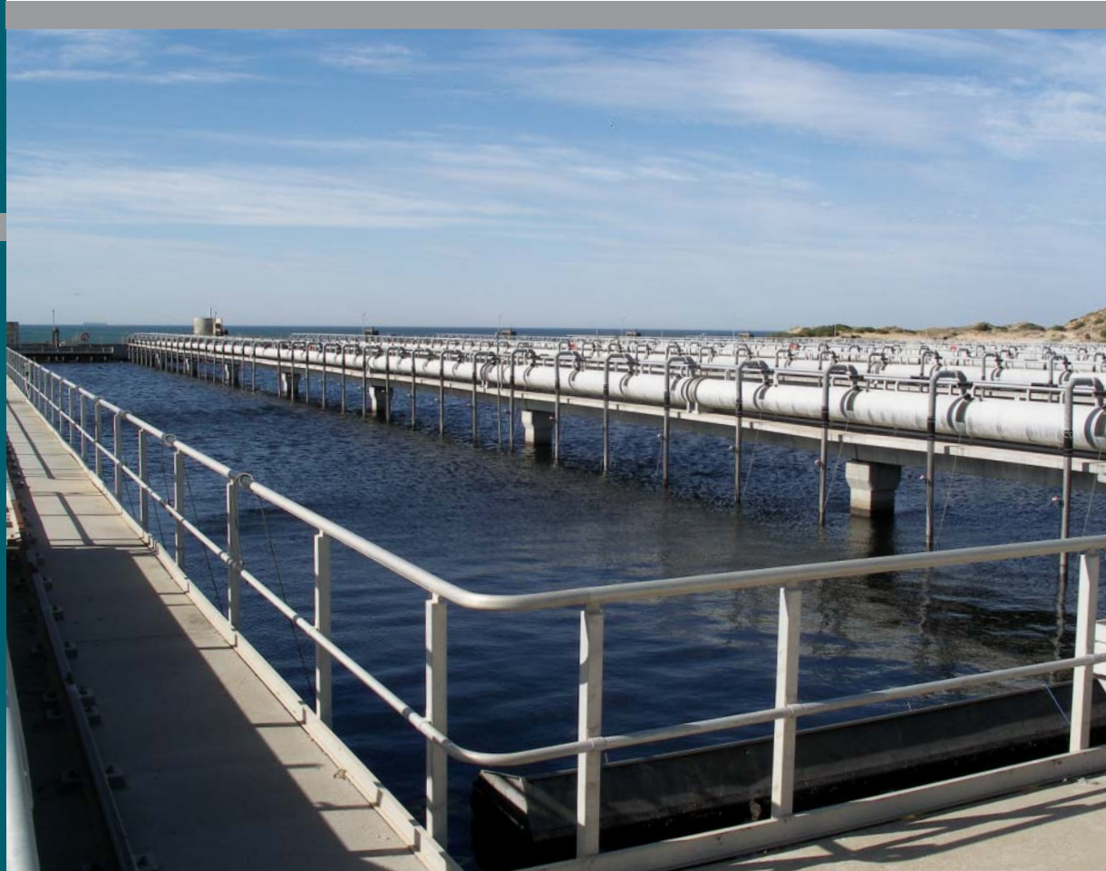
Black Rock Water Reclamation Plant, Barwon Water – Victoria
