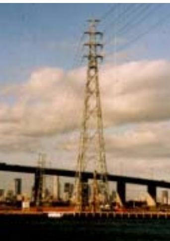
Power Transmission Towers
