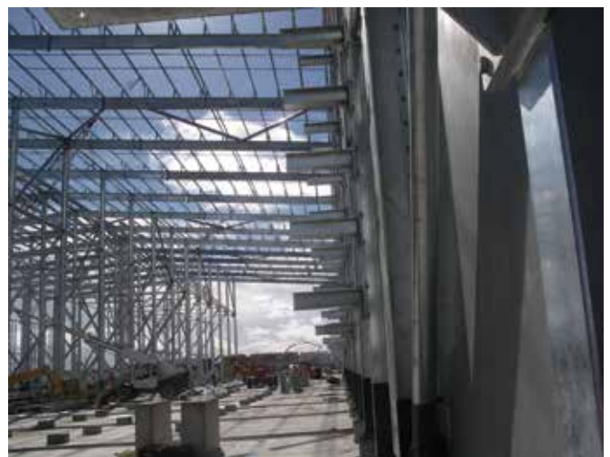
Sydney desalination plant.
